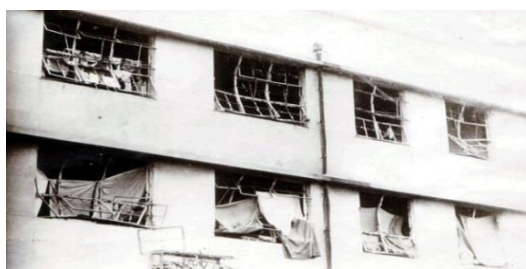
Window frames distorted inward by the blast
