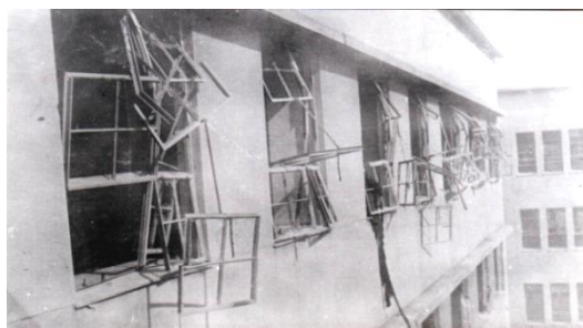
Window frames popped outward by the blast
